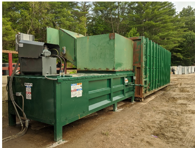
The new trash compactor is in place.
